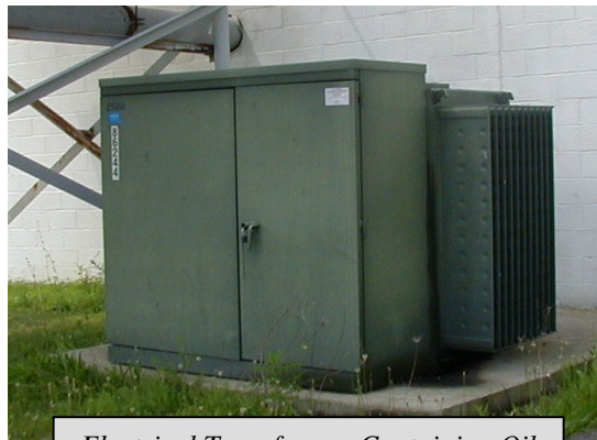
Electrical Transformer Containing Oil
