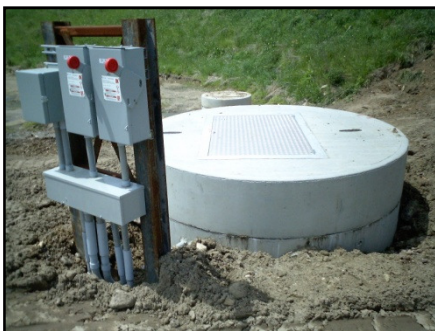
Treatment pumps transfer filtrate to oil-water separator
