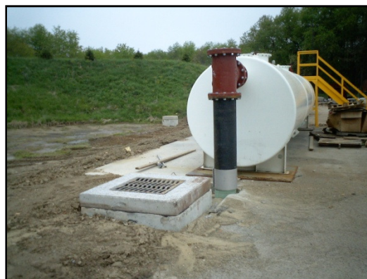
6,000-gallon oil-water separator
