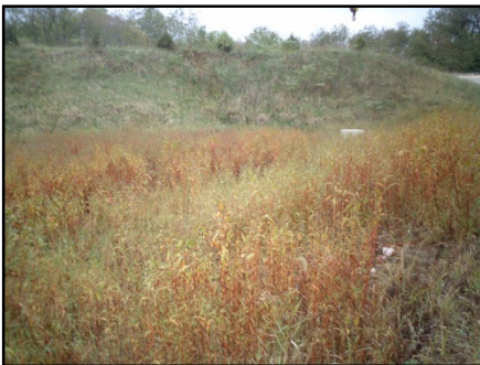
536,000-gallon detention pond
