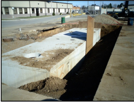
14,000-gallon underground collection tank
